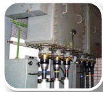
Power sensitive equipment
